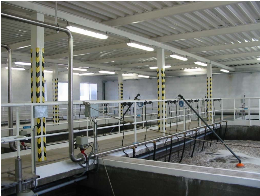
Biological wastewater treatment facility at the Kvasiny plant
